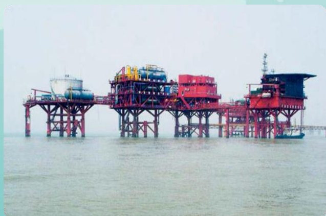
Offshore platform polymer injection Equipment
