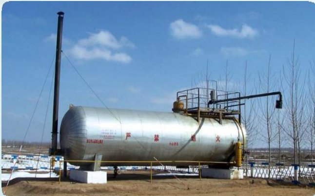
Oil Well Multi-phase Storage and Collection vessel
